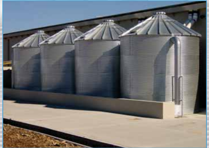
18,100 Gallons each (68,515 L) Water Storage Tanks for rain water collection
