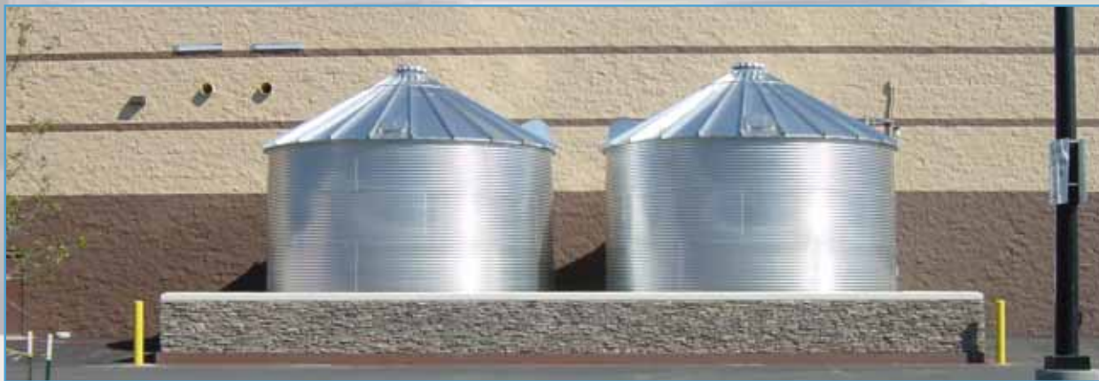
35,600 Gallons each (134,760 L) Water Storage Tank
