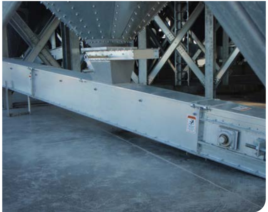
Hopper silos allow for easy clean-out.
