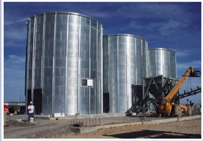
Open top Aggregate Silos are installed with wind rings to stiffen the top ring wall.
