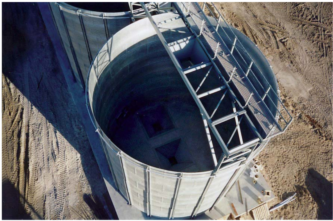
Aggregate silo showing discharge openings at floor level.
