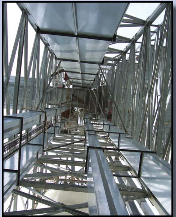
Equipment Support tower constructed with structural steel columns, beams and braces.
