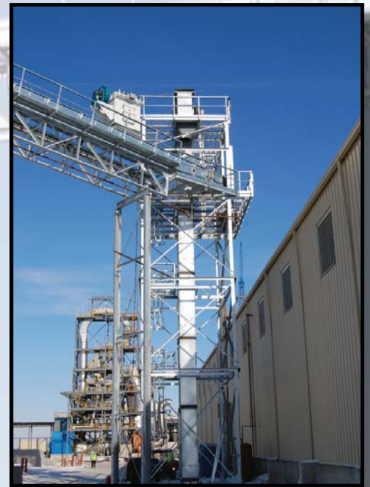
Our custom designs allow catwalks and equipment to connect at angles and inclines to suit requirement of the site.
