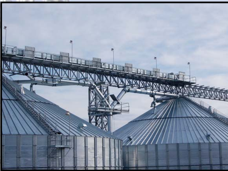
245' (74.68 m) long catwalks with 130' (39.62 m) clear span and 6' wide (1.83 m) wide Under-Truss with 10' (3.05 m) wide deck support designed for high capacity grain handling.
