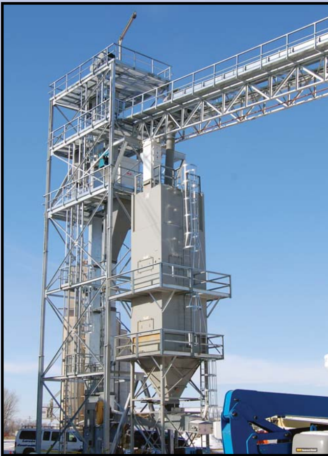
Custom catwalks and towers with top and intermediate platforms.
