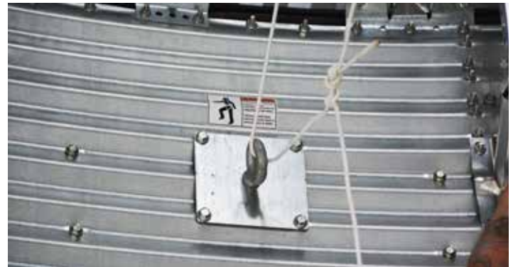
Anchor point installed below the roof inspection hatch
